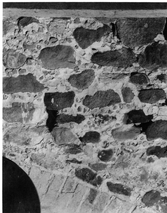
Fig. 4. Udsnit af murværket på østsiden af \dagger tårnets østmur (s. 3633). KdeFL fot. 1991. - Section of masonry from the western part of the church, presumably constructed around the year 1500 as a tower, but reduced early to its present state.
