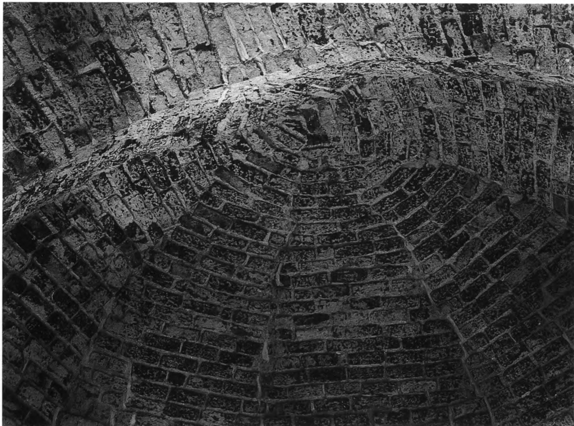
Fig. 96. Polygonalt hvælv i korsarmsende, afklædt under restaureringen 1917-21 (s. 3095). Mogens Clemmensen fot. - Polygonal vault at the end of transept, exposed during the restoration 1917-21.
