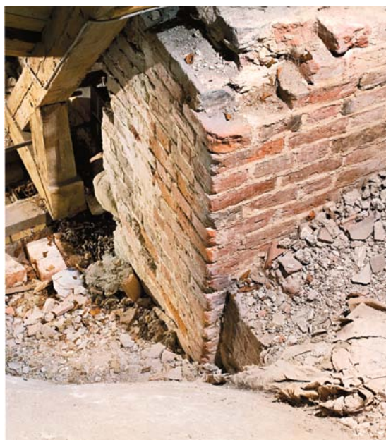
Fig. 23. Murforhøjelsen af den romanske kirke i sammenstødet mellem kor og nordre korsarm, set fra sydvest (s. 2116 ff.). Foto Arnold Mikkelsen 2008. – Heightening of the wall of the Romanesque church at the junction between the chancel and the north transept, seen from the south-west.
