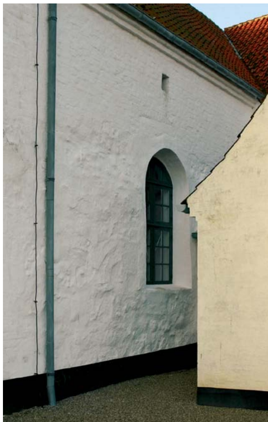
Fig. 117. Korets nordfacade, set fra nordøst (s. 2117 ff.). Foto Thomas Bertelsen 2009. – North facade of the chancel, seen from the north-east.
