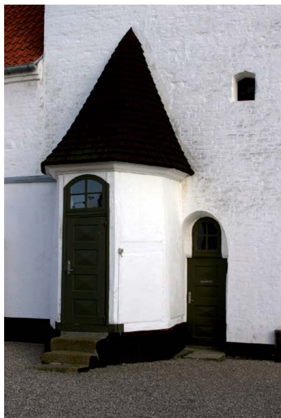
Fig. 19. Tårnets trappehus, set fra sydøst (s. 2115). Foto Thomas Bertelsen 2009. – The tower staircase, seen from the south-east.
