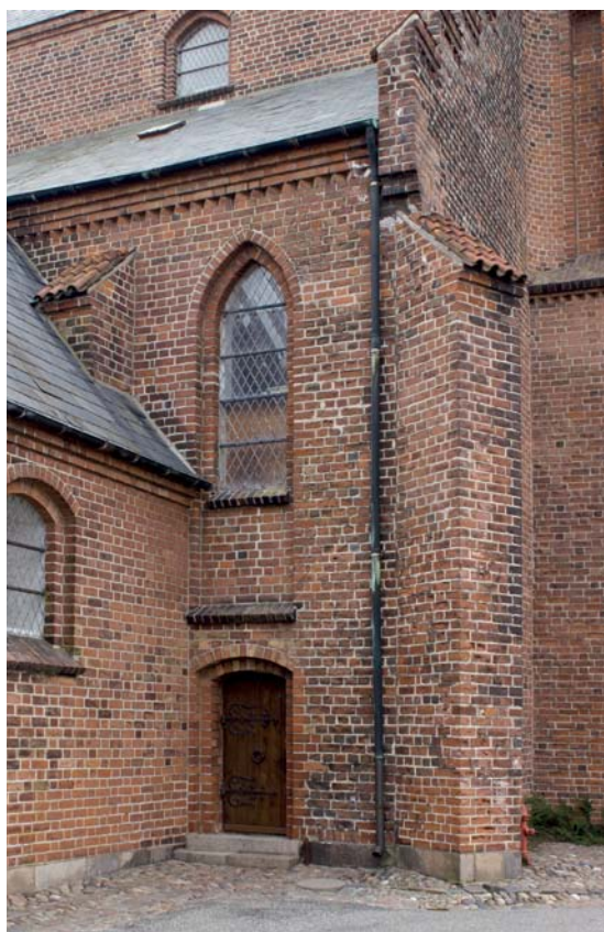
Fig. 36. Nordre sideskibs vestligste del, set mod sydøst. Foto Thomas Bertelsen 2011. – Westernmost part of the north side aisle, seen towards the south east.
