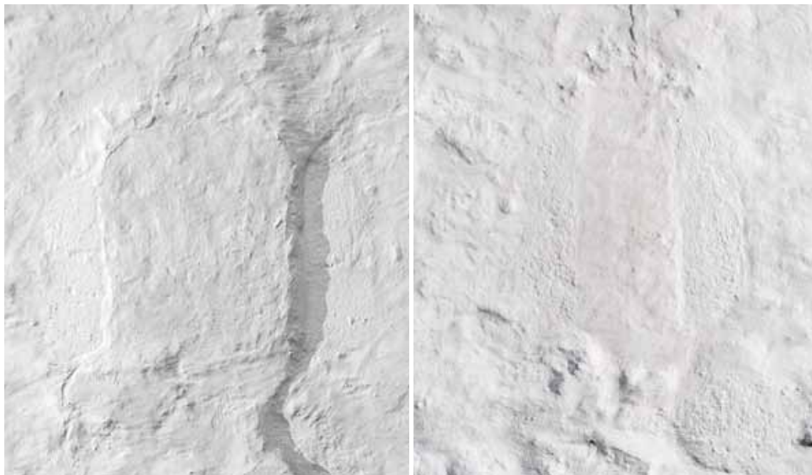
Fig. 5-6. Tilmurede vinduer i kirkens nordside. 5. Romansk? vindue i koret (s. 3311). 6. Romansk vindue i skibet (s. 3311). Foto Arnold Mikkelsen 2014. – Bricked-up windows in the north side of the church. 5. Romanesque? window in the chancel. 6. Romanesque window in the nave.
