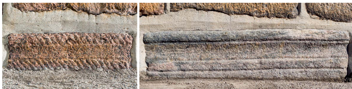
Fig. 7-8. Kragsten (s. 4197) indmuret i soklen under skibets sydside. Foto Arnold Mikkelsen 2016. – Corbels walled into the base beneath the south side of the nave.
