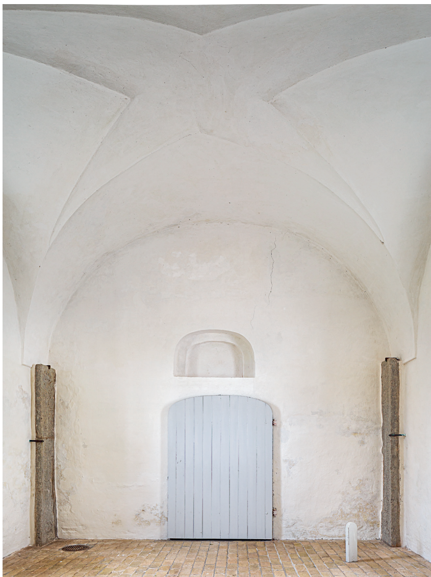
Fig. 15. Sydkapellets indre set mod syd (s. 5784). Foto Arnold Mikkelsen 2019. – The interior of the south chapel looking south.
