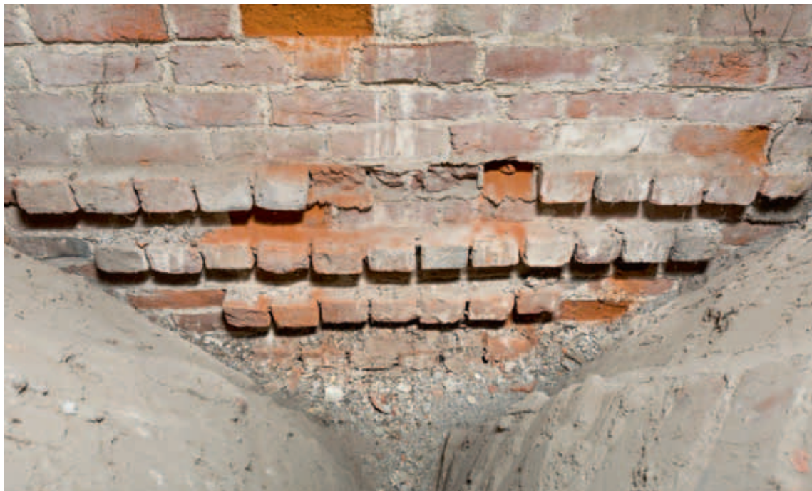
Fig. 23. Hvælvfortanding øverst i korets sydvæg, set fra loftet mellem de to hvælv (s. 1376). Foto Arnold Mikkelsen 2015. – Vault toothing at top of south wall of chancel, seen from the ceiling between the two vaults.
