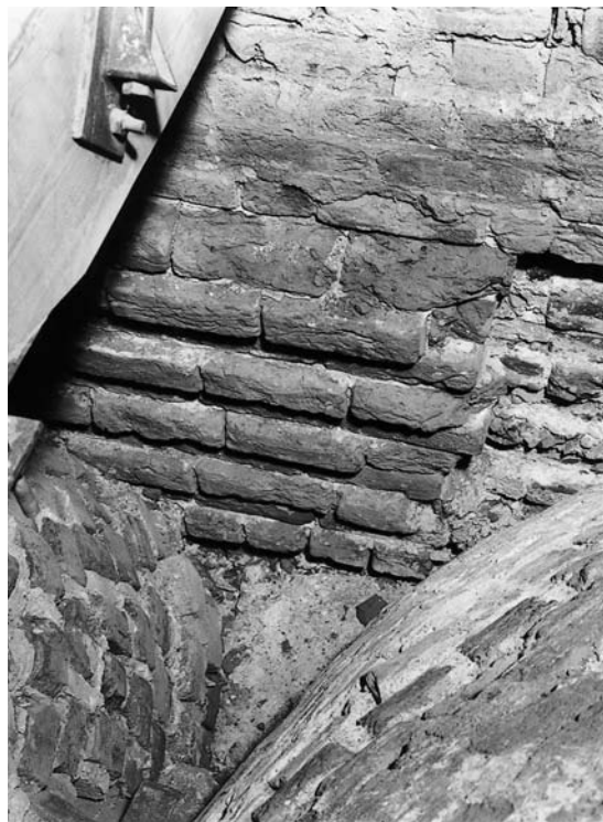
Fig. 18. Hvælvfortanding øverst i skibets nordvæg, set fra loftet mellem 2. og 3. hvælvfag (s. 95). Foto AM 2004. – Vault tothing at the top of the north wall of the nave, viewed from the ceiling between the second and third bay.
