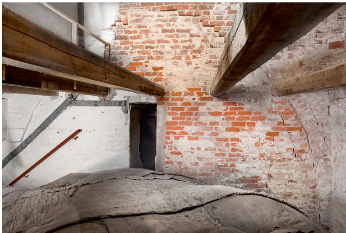
Fig. 13. Skibets vestre, ommurede gavlvindue med buestik set fra vest (s. 24596). Foto Arnold Mikkelsen 2016. – Rebuilt western gable of nave with relieving arch, seen from the west.
